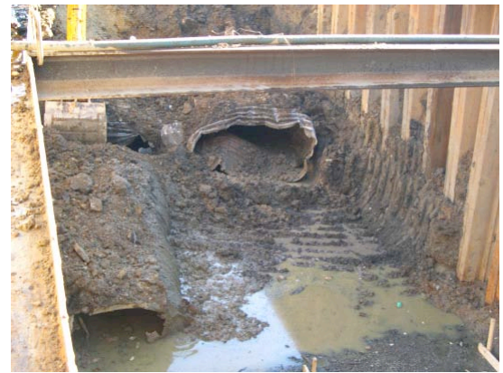
Storm water Interceptor Failure
