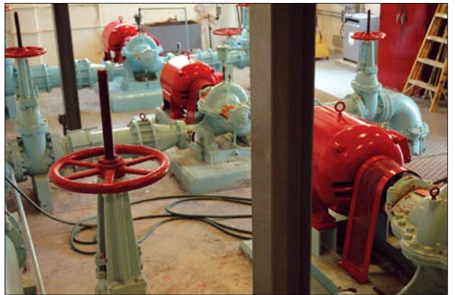
Five water pumping stations like this one are located around Arlington. The pumps turn on when needed to send water to higher elevation tanks or reservoirs.
