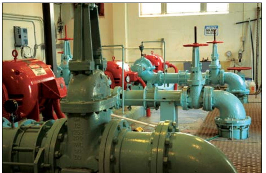
Pumping stations such as this one have as many as four pumps that serve as backups and assist in pumping a higher volume up to the water tower when levels drop below 25 feet.
