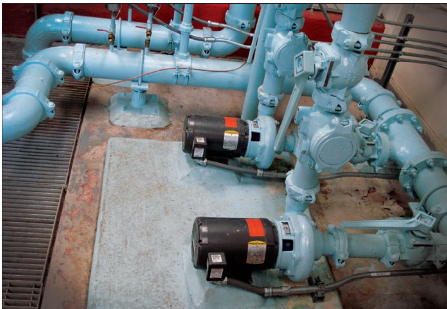
Installed in 2009, these booster pumps at Arlington's Minor Hill facility provide improved water pressure to the surrounding area.
